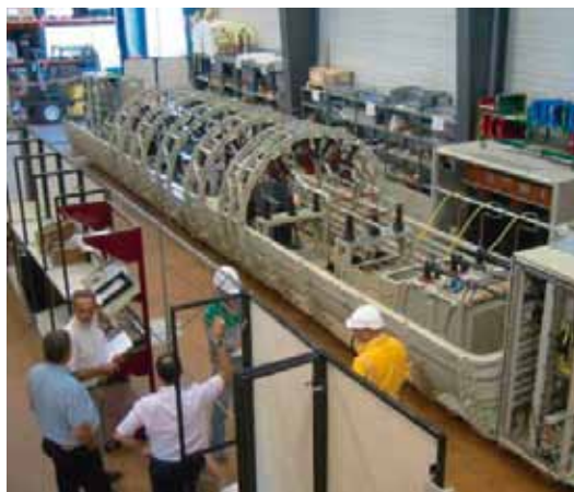
| Circuit breaker module rack for the Ormen Lange pilot station
