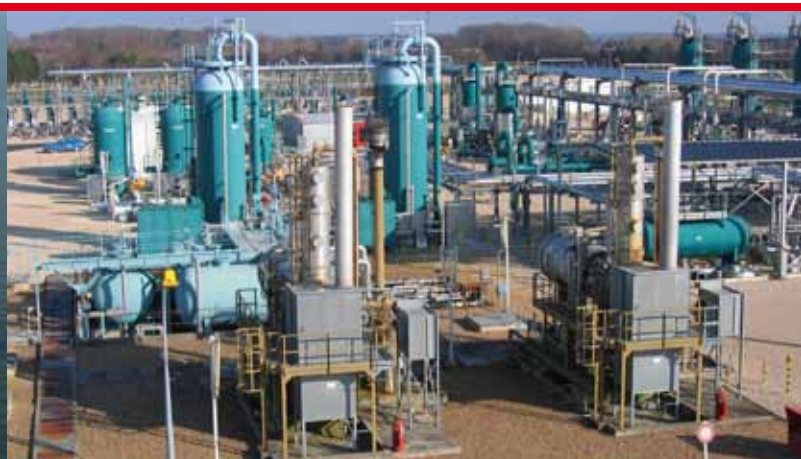
| GDF-SUEZ Chémery gas storage station
