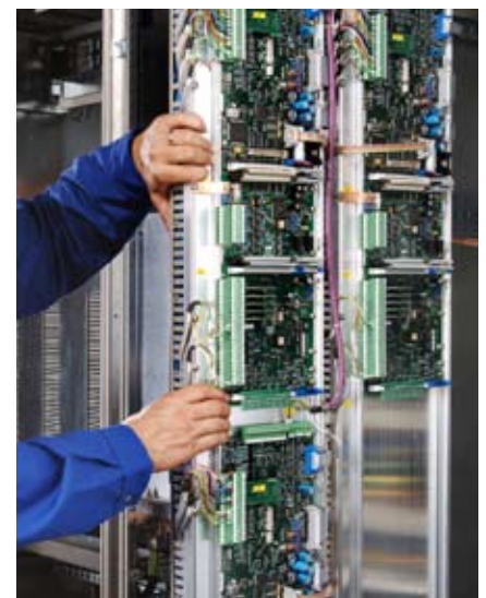
Control unit on slide out runner
