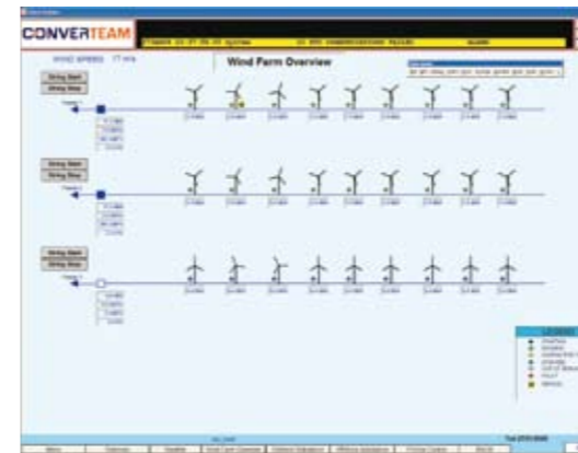
Control/monitoring system – wind farm overview
