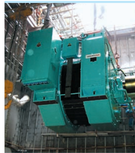
11 MW - 514 rpm diesel & gas engine-driven generator
