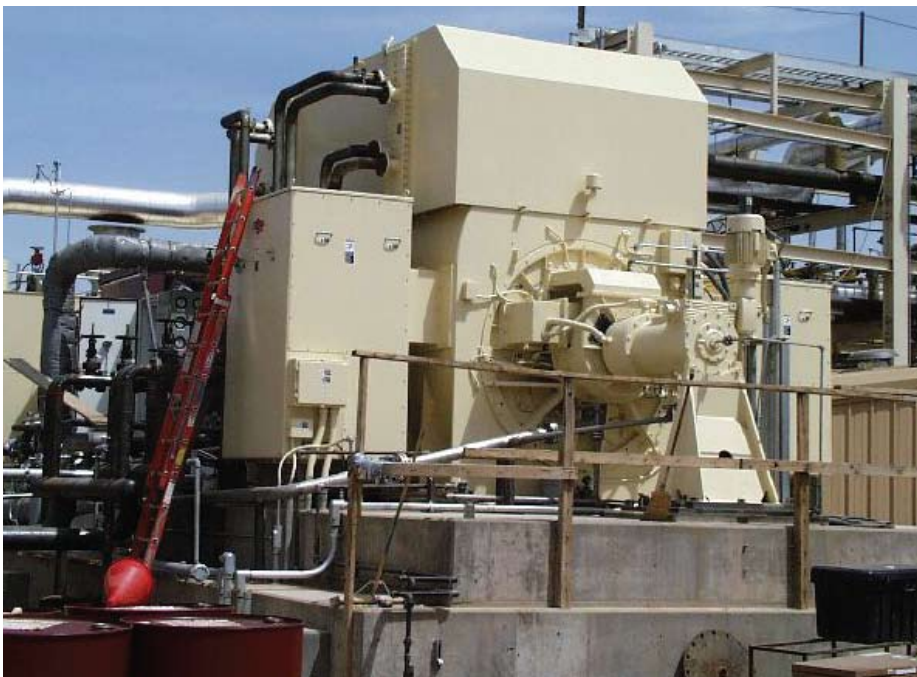
2-Pole Generator with TEWAC enclosure in a utility generating station.
