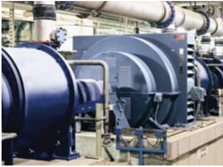
Vacuum pump drive
