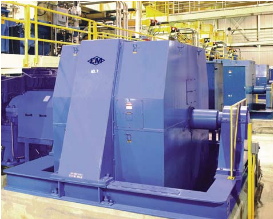
Synchronous motor driving a grinder in a paper mill.
