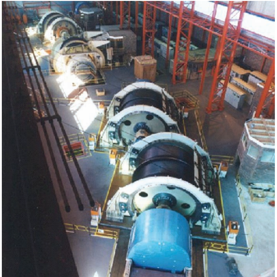
View of both 7.4 MW Induction Motors and Drum Winders electrically coupled together
