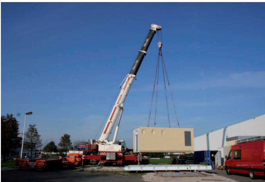
ConverSOL power system supplied as a containerised solution
